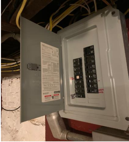
Example of an electrical panel (interior)
