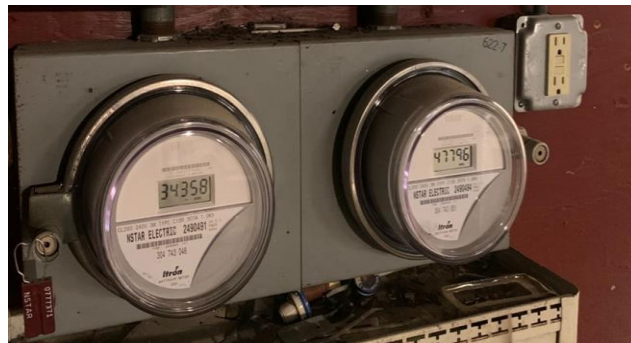
Example of an electrical meter
