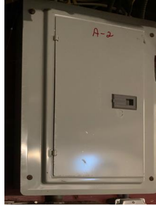
Example of an electrical panel (exterior)
