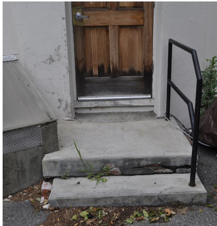
THE ARMORY Stoop deterioration
