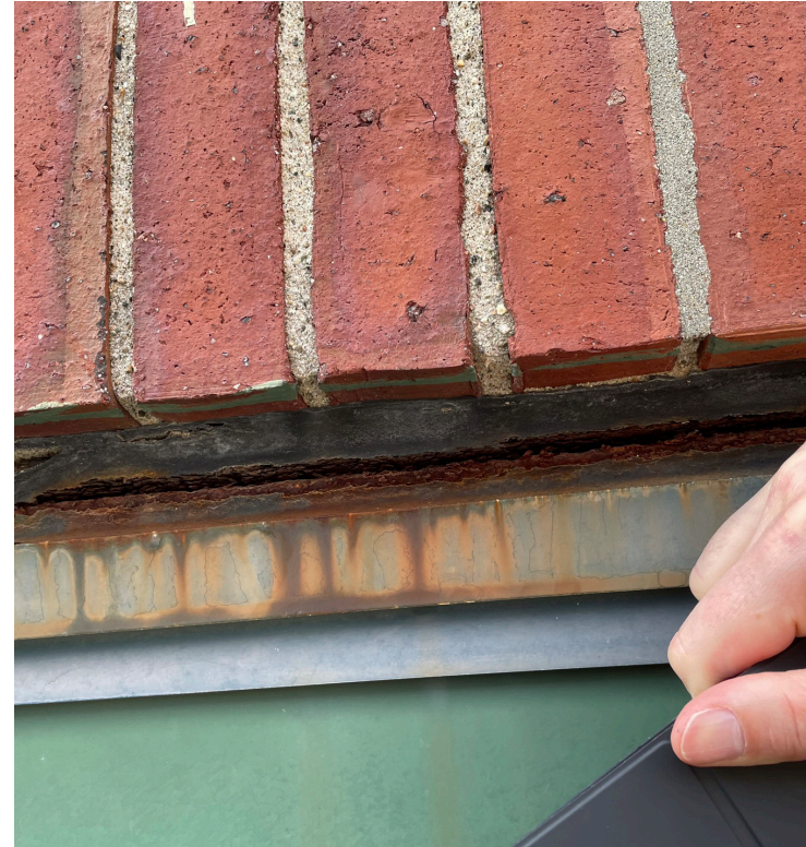
EDGERLY Corrosion of window lintels
