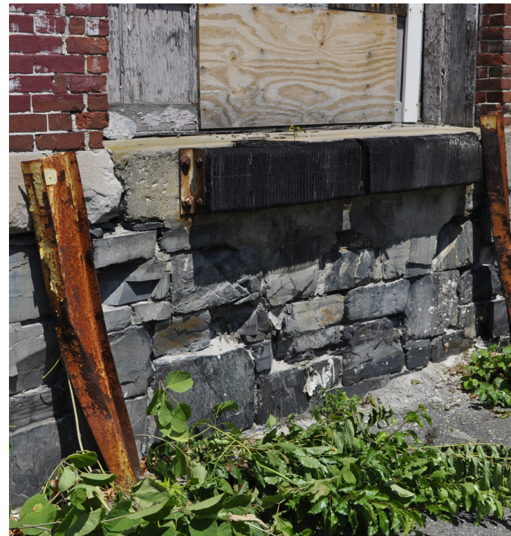
24 CROSS STREET EAST Deteriorated foundation
