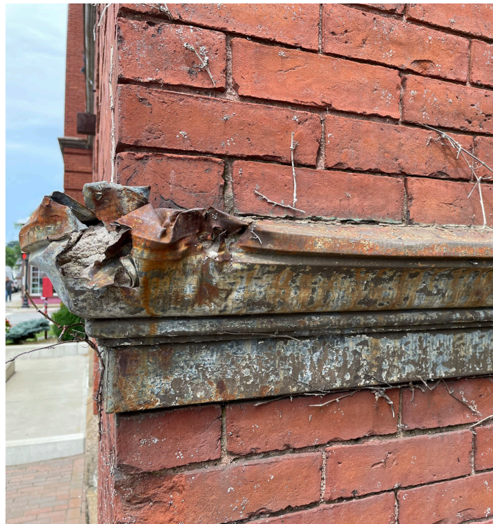
165 BROADWAY Damaged Cornice
