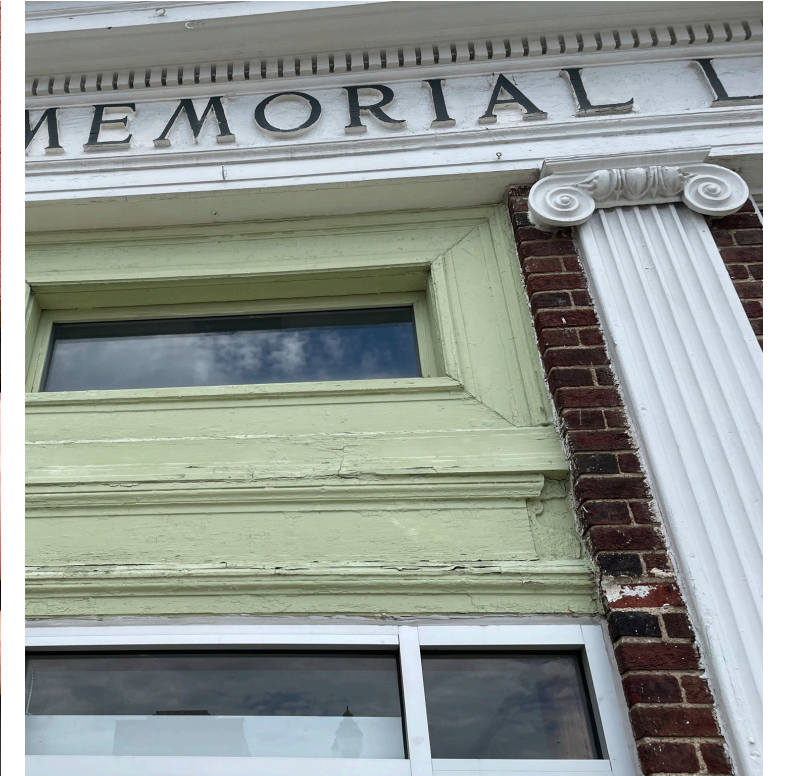
115 BROADWAY Weathering of exterior millwork
