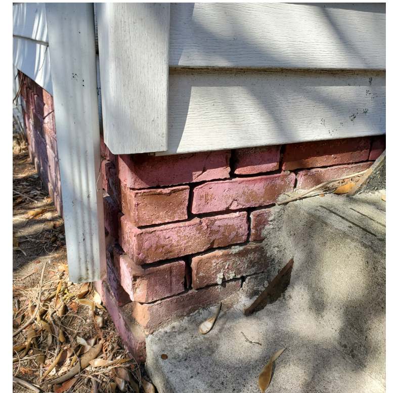
45 COLLEGE AVENUE Deteriorated foundation
