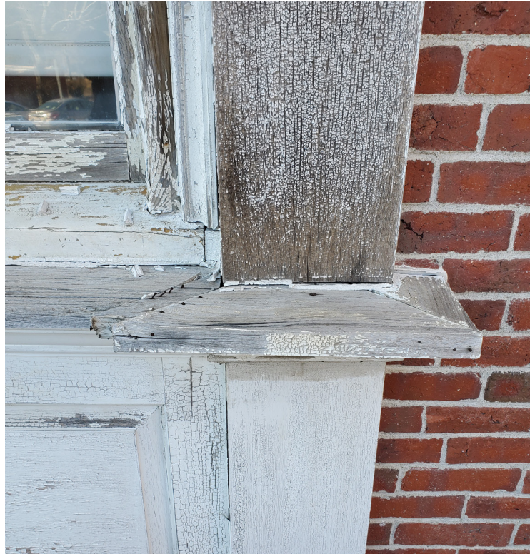
CITY HALL Deteriorated exterior wood trim
